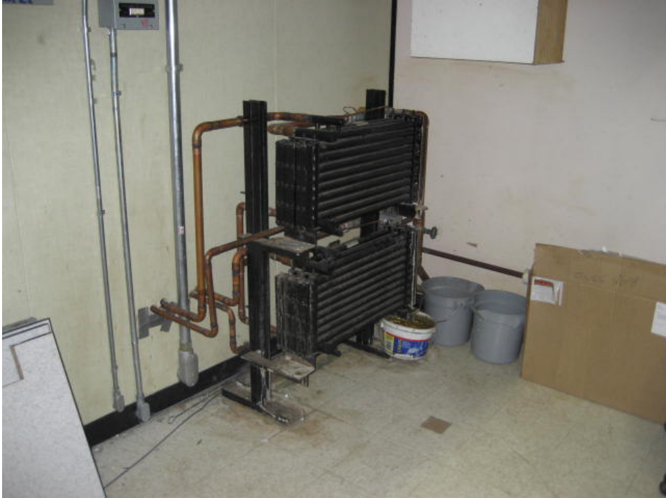
Photo 3: Existing IT Server Room AC Unit Water Cooled Condensing Unit
