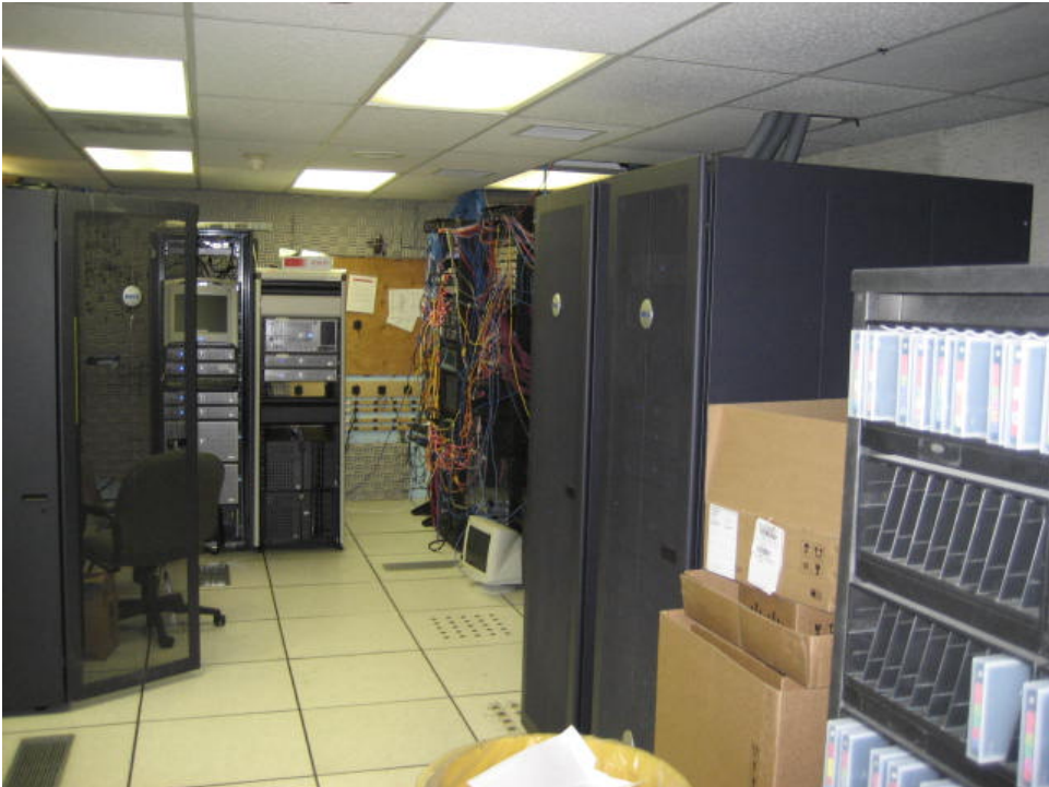
Photo 2: IT Server Room
