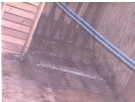
Pic #5 Hose Hanger area rot/deterioration
