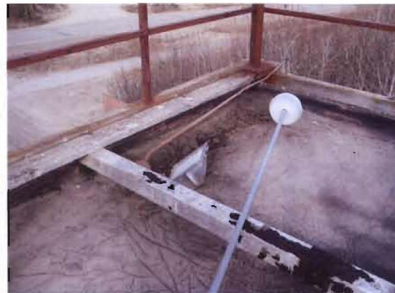
Pic #6 SW Roof area (5' slump under light)
